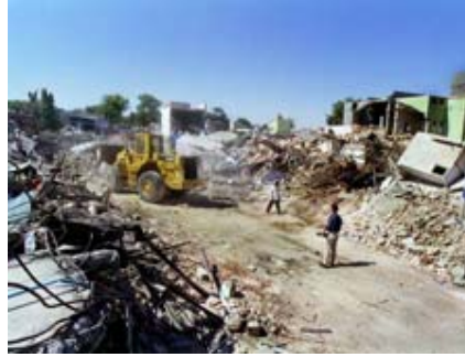
Figure 4.27 Clearing rubble after an earthquake, Bhuj, India
