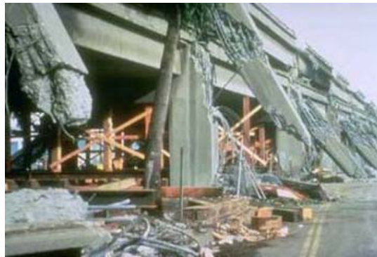
Figure 4.28 Collapsed bridges – USGS
